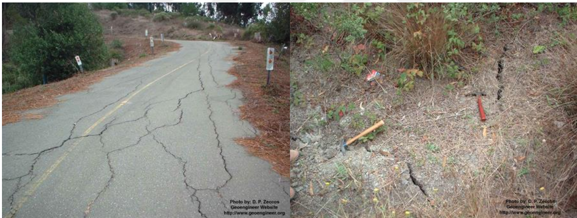
Figure 1.8. Cracks due to expansive soil (URL-1, 2021).
